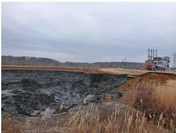
Figure: The Dan River Steam Station Ash Pond Post-Failure Source: EPA Region IV Pollution Report via Wikipedia.
