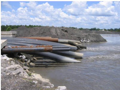
Figure: Wastewater discharge location for the Barry Electric Generating Plant near Bucks, AL (Source: Alabama Public Radio via EPA)
